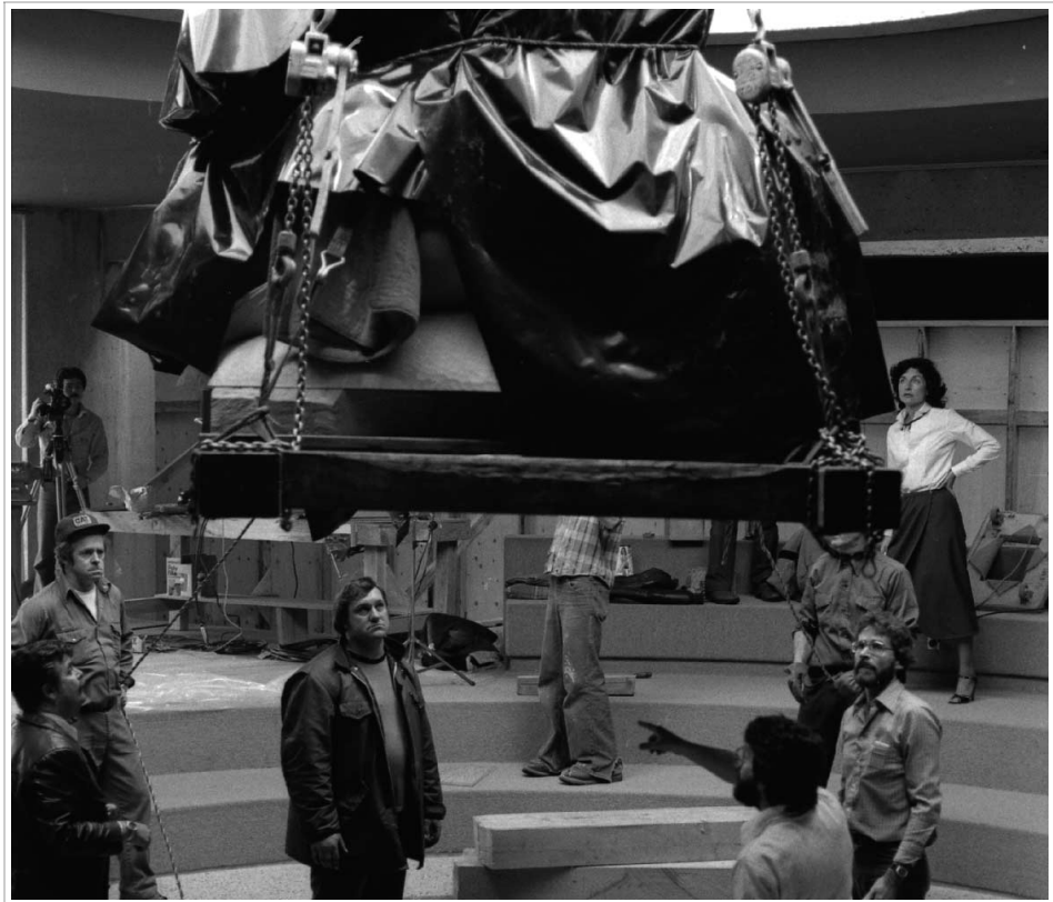
Bill Reid's The Raven and the First Men is lowered through the skylight for installation on what was once gun emplacement number two. MOA Archives: William McLennan fonds, a043191. Photographer unknown, ca. 1980.
