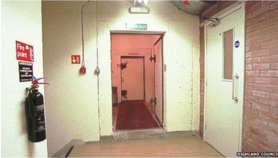
Inside Highland Council's Raigmore bunker in Inverness
