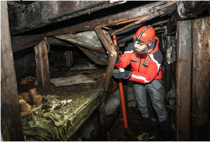
The inside of a cave being restored in the Stelvio Pass area. The structure dates back to 1915. (Courtesy of Giovanni Cadioli)
