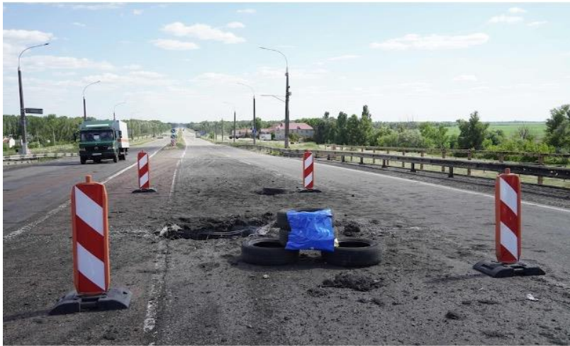
Craters on the Antonovskiy Bridge over the Dnieper River as a result of poorly weaponized rocket strikes – minimum damage and quickly fixable. AFP/Getty.
