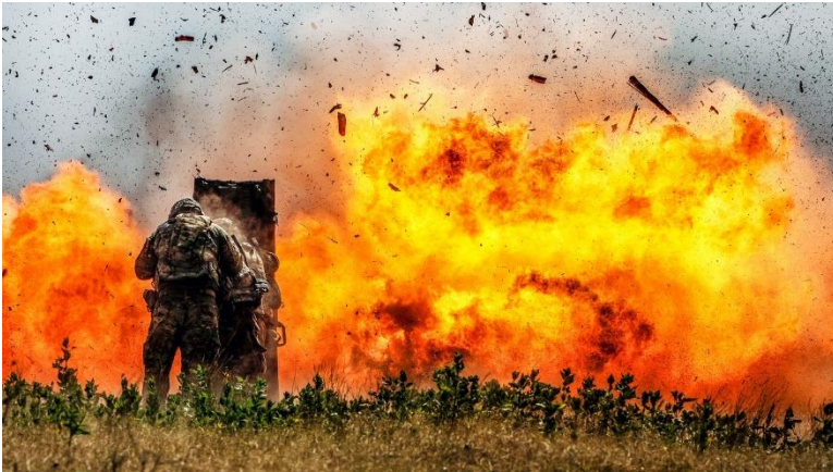
Combat engineers from the 2 nd Armored Brigade Combat Team, 1 st Cavalry Division blast through a concrete wall during demolition training at Curry Demo July 17.
